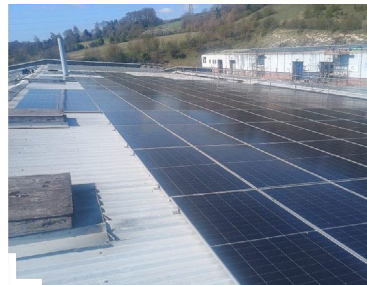
Solar panels at our High Wycombe facility.
